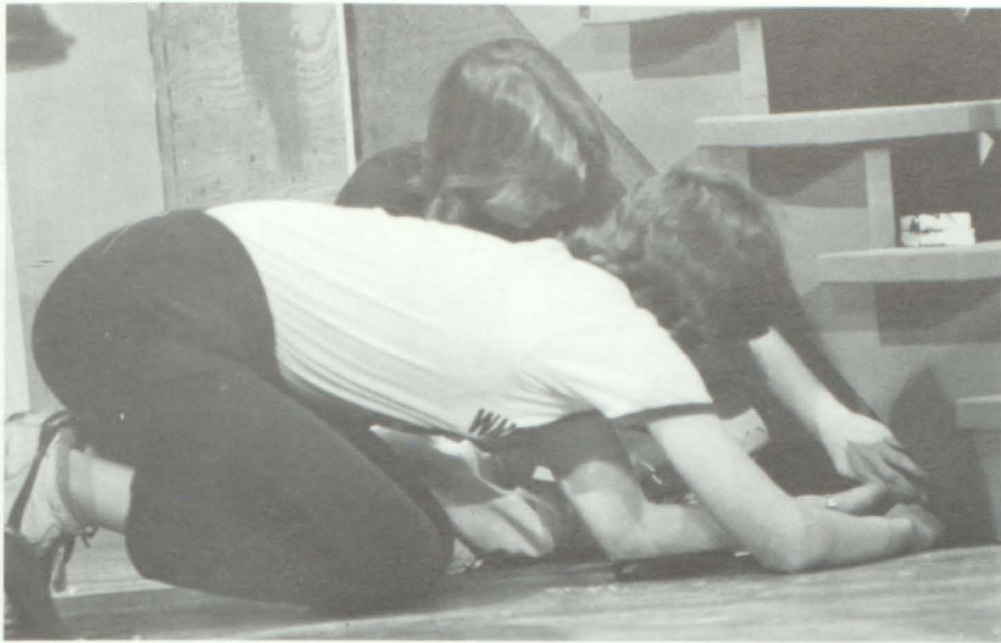
Two set crew members, Jo Swem and Stephanie Cooley , work intently on preparing the stage for the opening night.
